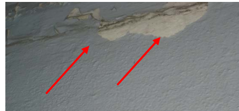
Photo 4. Asbestos-containing exterior wall texture is located on the east wall of the custodial supply area #1 and the custodial common area of the structure.
