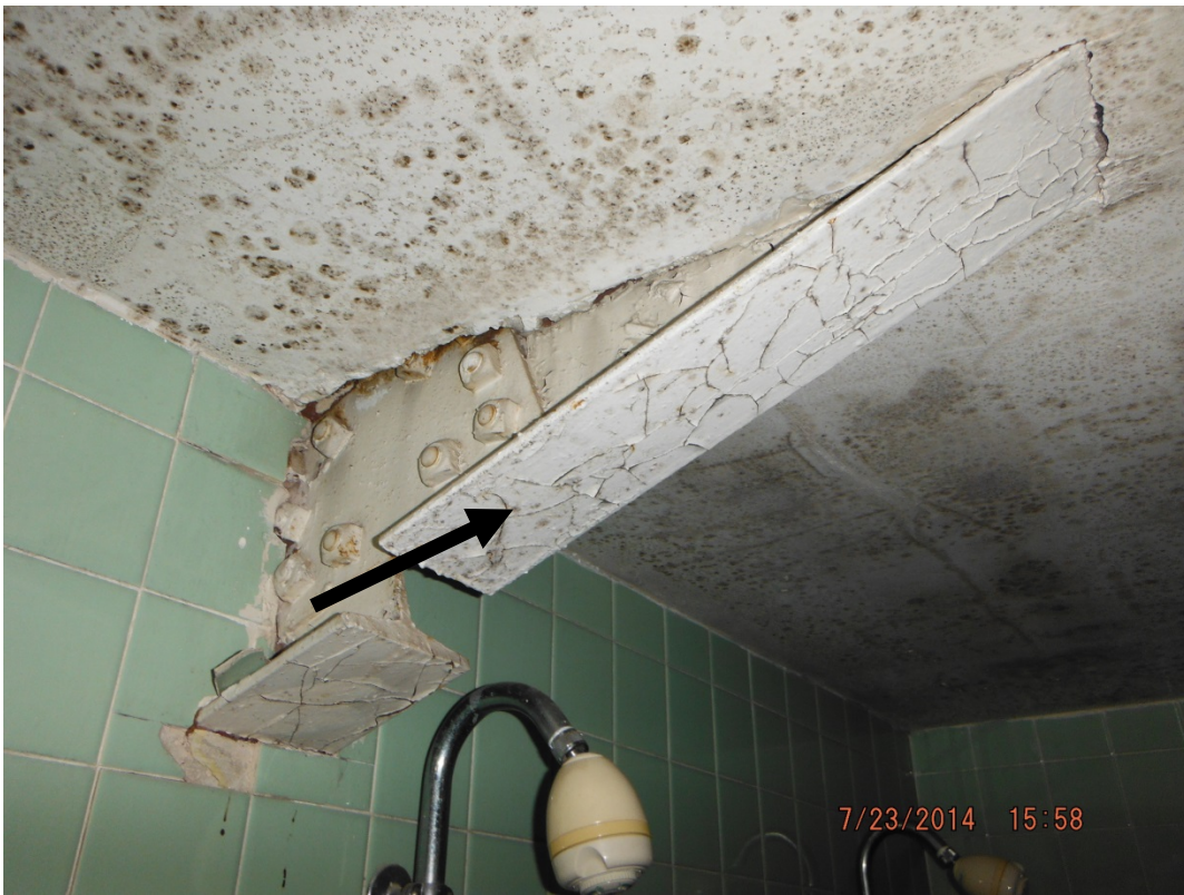
Lead-based paint on structural steel in shower
