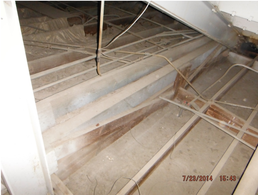
Lead-based paint on wooden joist from previous structure on top of existing structure
