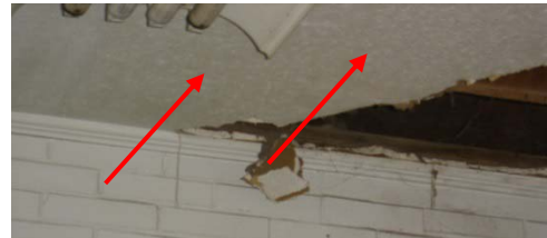
Photo 2. Asbestos-containing spray-applied ceiling texture located in various rooms of the structure.
