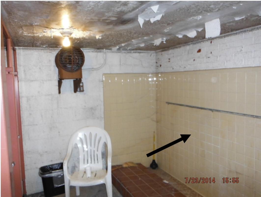
Lead in ceramic yellow tile by urinal in the bathroom
